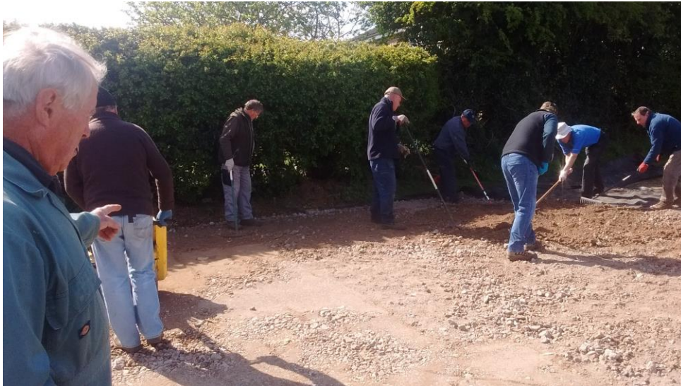
Working with FSALG to lay the groundworks for a new car parking area at the Ferry Road allotment site.
