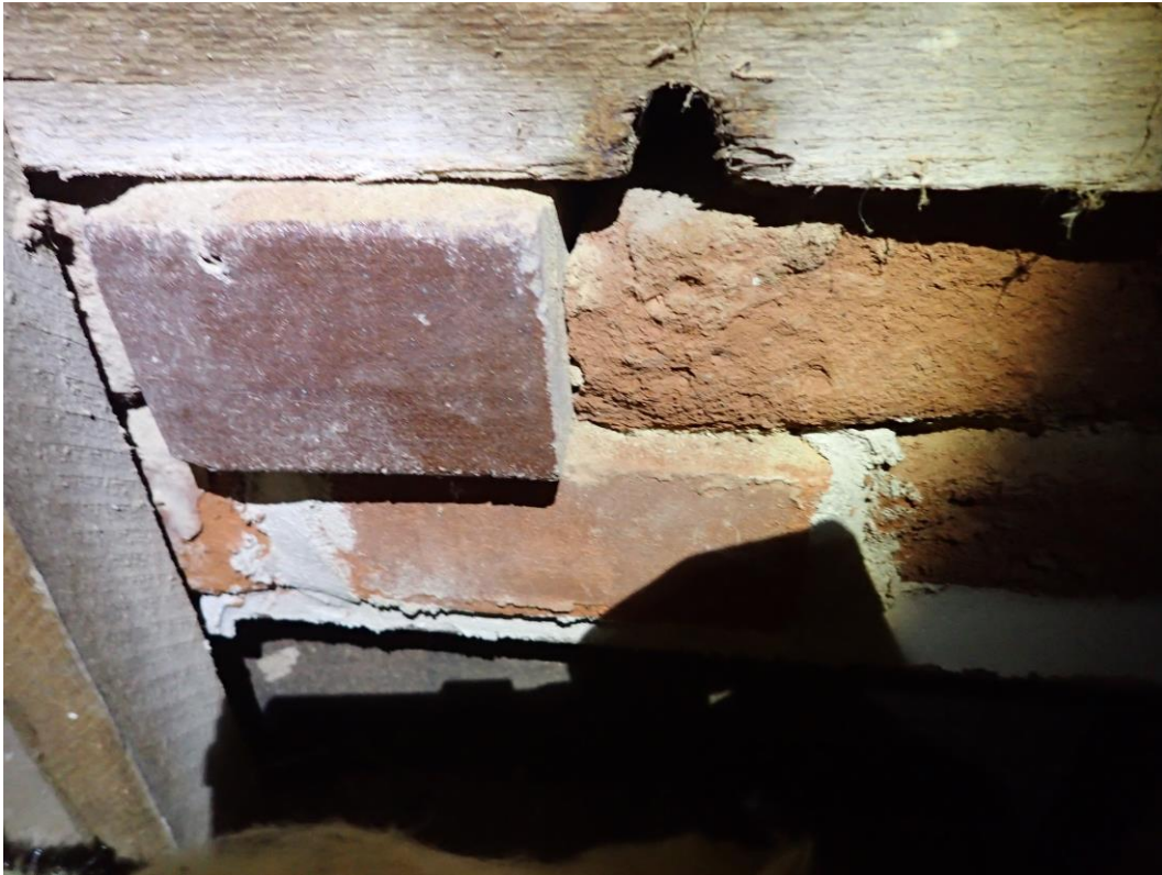
BRICKWORK OVER RSJ LINTEL HAS BEEN MADE GOOD WITH FRESH LIME MORTAR POINTING.
